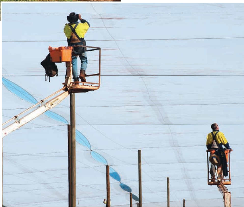
Above: Contractors work feverishly to install the remaining 38 hectares of protective canopy from Net Pro.
