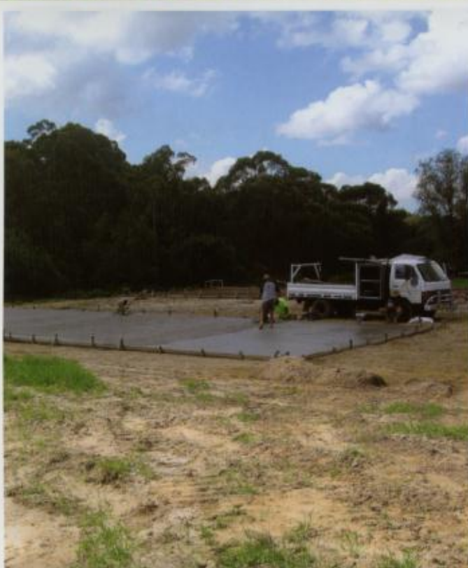
When complete, the facility will include two propagation greenhouses with concrete floors.
